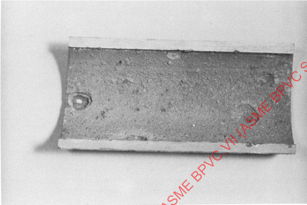
Figure 200.5.2-1 Oxygen Corrosion in an Economizer Tube
